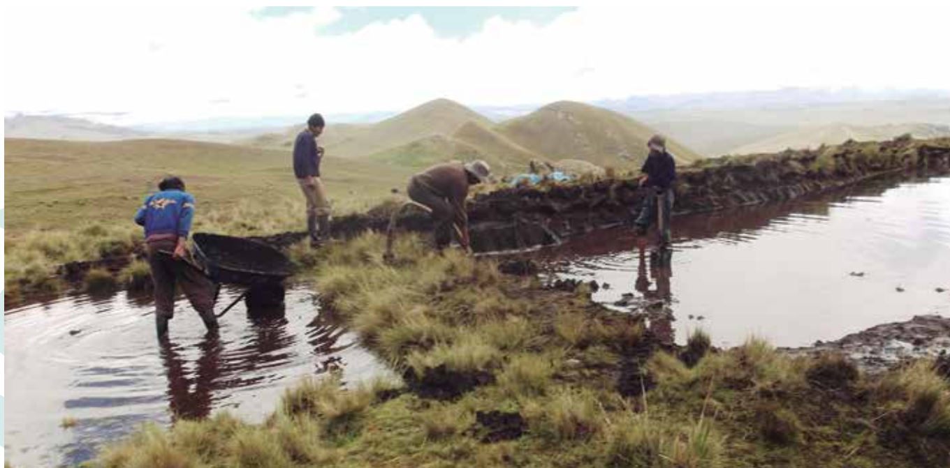
Farmers in Huacrahuacho micro-watershed (Cusco) building a dyke of the water reservoir.
